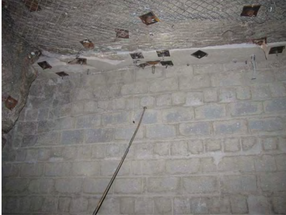
Figure 5. Surface spalling at the top corner of the explosion wall in the intake drift of Panel 1 during February 2012.
